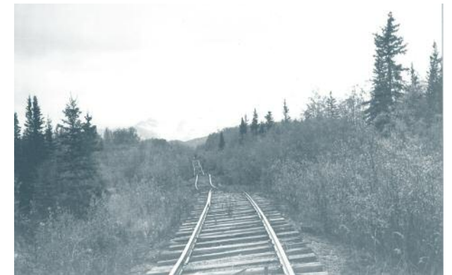
The abandoned Copper River and Northwestern Railway near Strelna in south-central Alaska illustrates how building a railroad on permafrost thaw can cause the railroad bed to settle unevenly. Although maintenance and use of the railroad was halted in 1938, lateral displacement continues today. (Image courtesy of U.S. Geological Survey)
