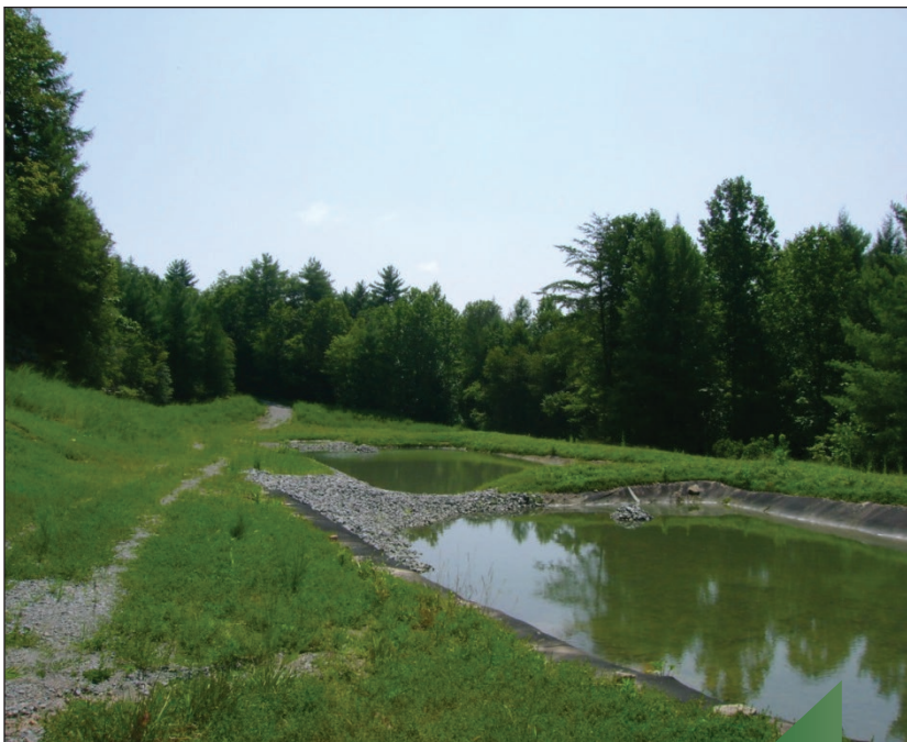
A variety of treatments installed in the Crab Orchard Creek watershed in Morgan County, Tennessee, helped reclaim the abandoned coal mine land and restore water quality.
