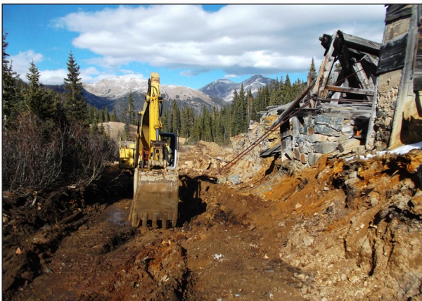
Removal of tailing piles around a historic mill structure in Summit County, Colorado.
