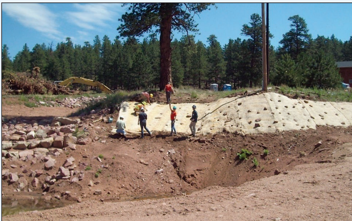
Erosion control mats were installed after a wildfire in Waldo Canyon in central Colorado.
