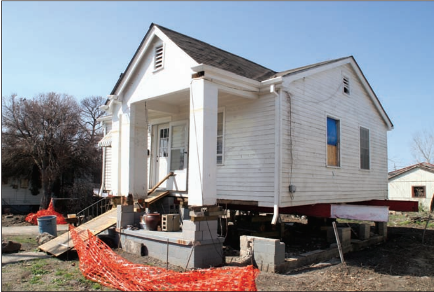
New Orleans, LA, March 8, 2006 – This house in Gentilly is in the process of being elevated above the base flood elevation adopted by the community in result of flooding from Hurricane Katrina. The homeowner will raise the house a total of 11' and has received the Increased Cost of Compliance (ICC) benefit included with his National Flood Insurance Program (NFIP) policy because of his compliance to the community's floodplain management ordinance. Robert Kaufmann/FEMA
