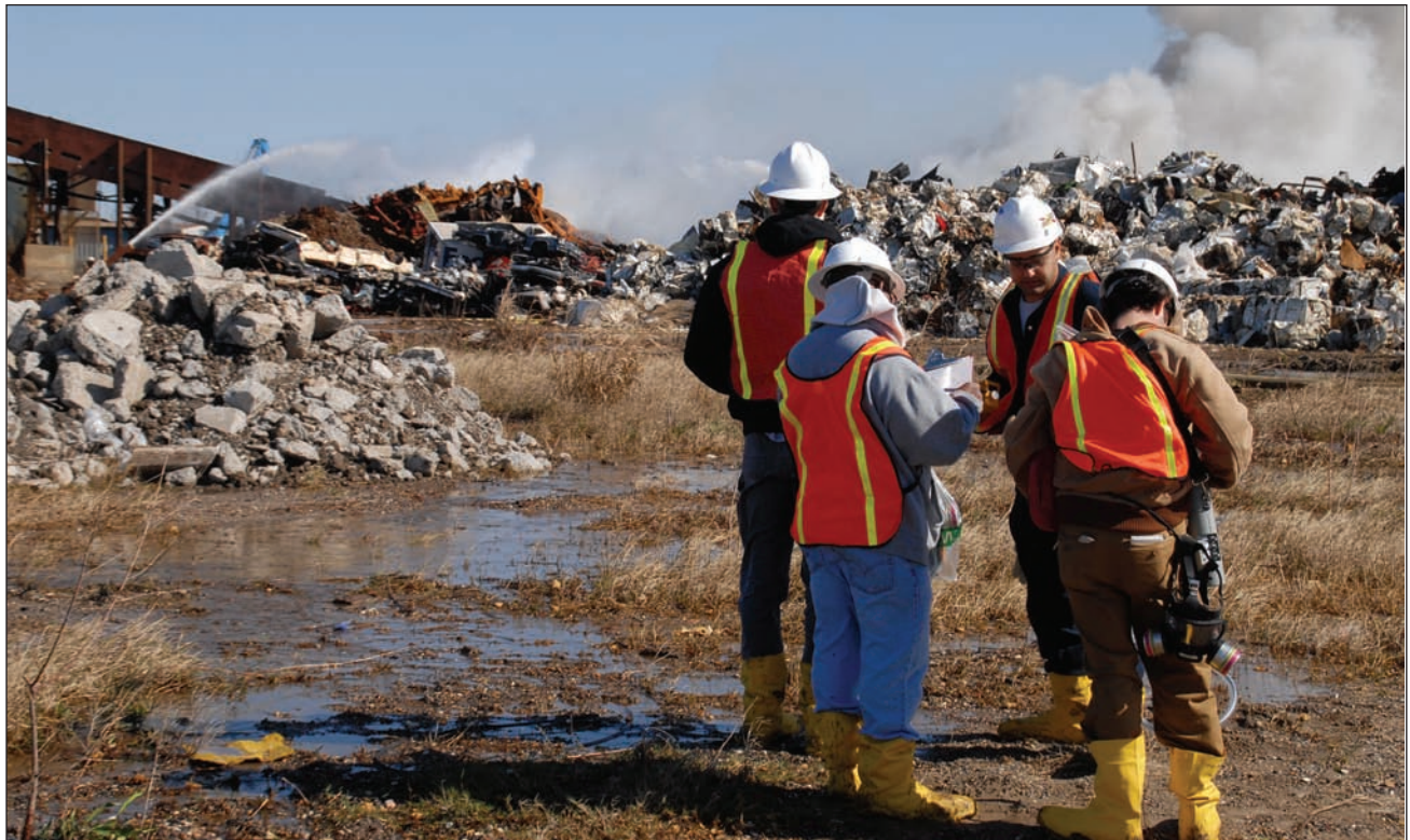
New Orleans, LA, 1-13-06 – Workers from the EPA were on the scene helping the New Orleans Fire Department when a fire broke out at this Hurricane Katrina debris processing plant. The EPA, funded by FEMA, are working to identify, monitor, and clean up any hazards. MARVIN NAUMAN/FEMA photo
