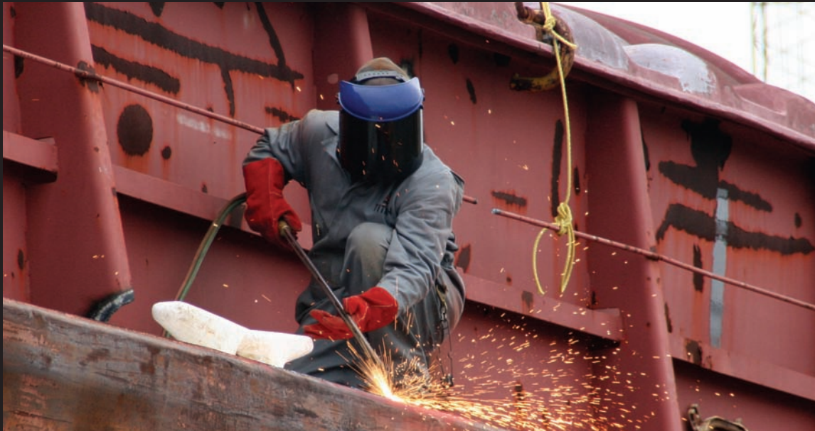
New Orleans, LA, February 24, 2006 – Dismantling of the barge grounded at the levee break in the lower 9th ward has begun as FEMA continues debris removal in this area. Robert Kaufmann/FEMA
