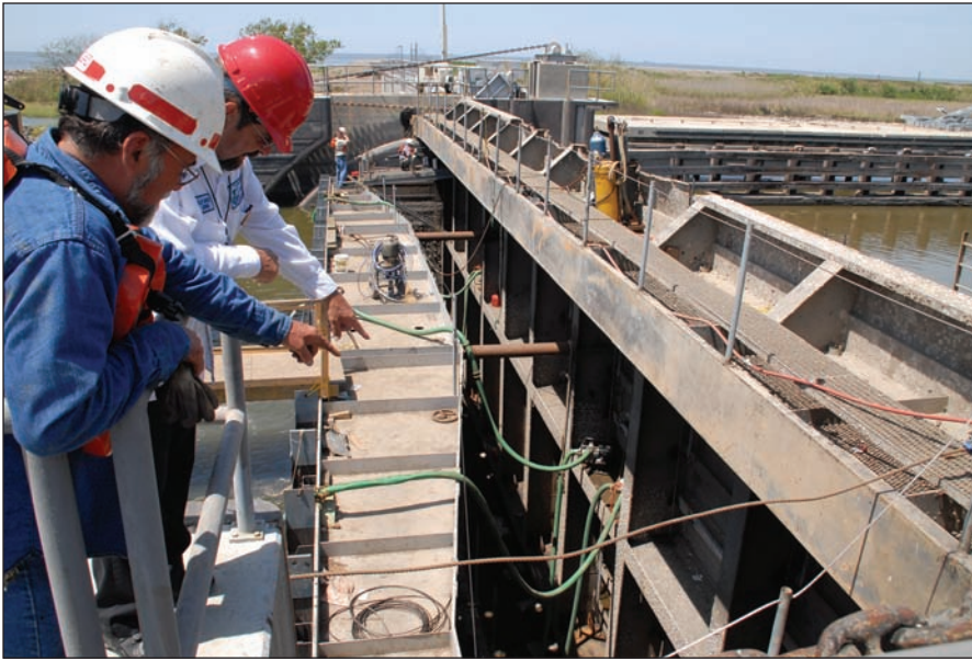
Empire, New Orleans, LA, 4-14-06 – U.S. Army Corps of Engineer Herbie Petit and Plaquemines Parrish Flood Gate Operator John Machella point to some pumps used to pump water out from between a temporary coffer dam and the Flood Gate so repairs can be made. FEMA is helping the Parrish government repair the Flood Gate that was damaged by Hurricane Katrina under its Public Assistance Program. Marvin Nauman/FEMA photo
