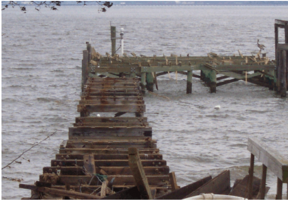
Figure 1-4. Damage to Gloucester Point, VA water level station.
