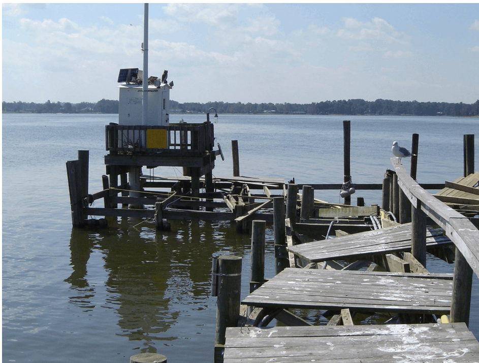
Figure 1-3. Damage to Lewisetta, VA water level station.
