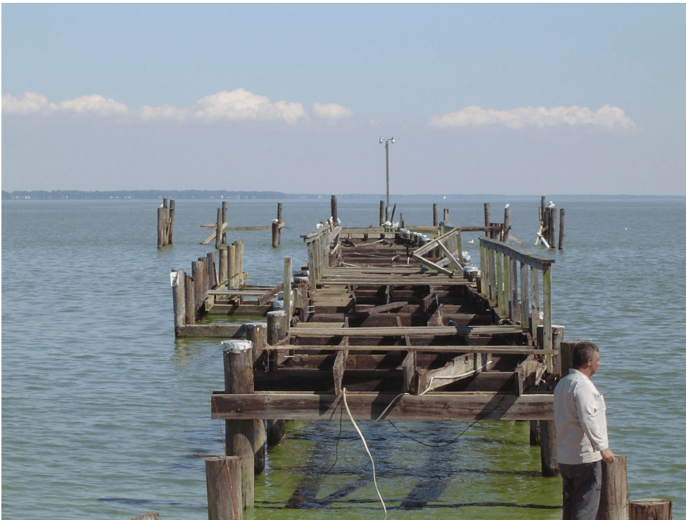
Figure 1-5. Damage to Colonial Beach, VA water level station.
