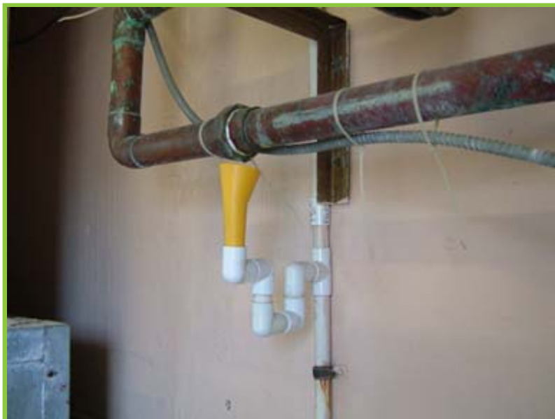
How not to repair a leak (actual example taken in the field).
