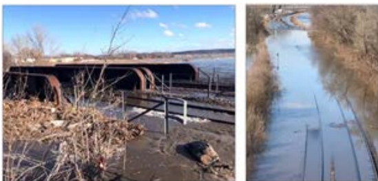
Flooding near Arlington, Nebraska
