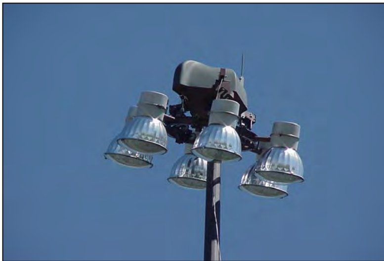
Figure 30. Misaligned Luminaire Ring.
