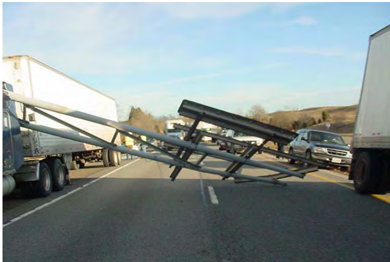
Figure 1. Cantilever Sign Structure Failure.
