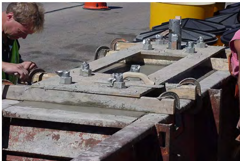
Figure 14. Template Secured to the Forms to Ensure Proper Alignment. Note Anchor Rod Threads Taped to Prevent Contamination by Concrete.
