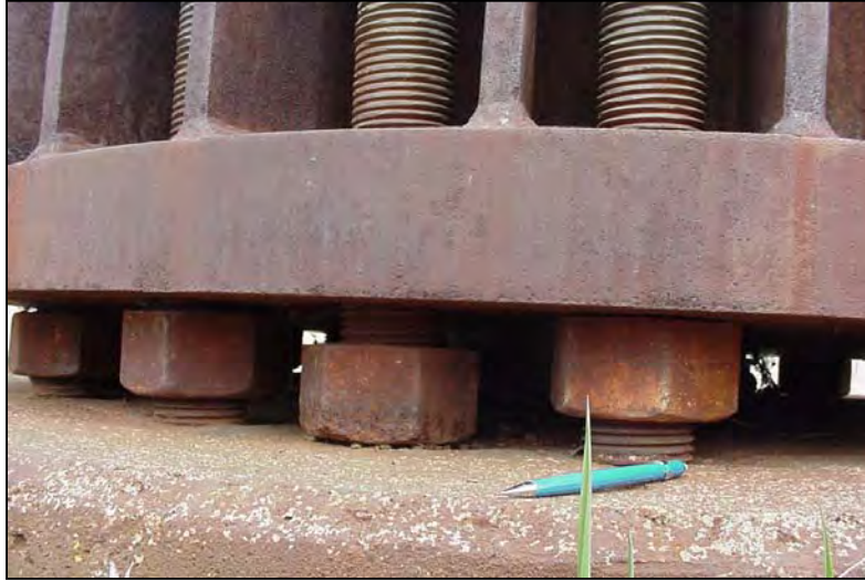
Figure 28. Loose Leveling Nuts on a High Mast Structure. (Note: Top Nuts on Chairs Out of Photo)
