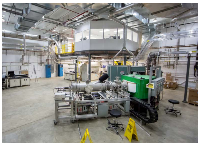
Figure 13: The EMIS 10 mA prototype inside of the upgraded host facility (Dec 2014)
