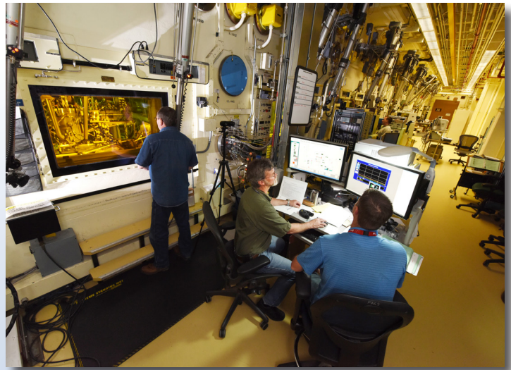
The main hot cell is 70 by 30 feet with 15 workstations each at a 4-foot-thick window.
