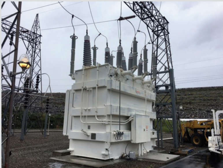
A new transformer at Folsom Dam was installed after periodic maintenance and Asset Management data indicated the old unit was reaching the end of its service life.
