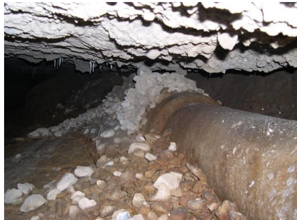
Loss of Foundation beneath Spillway Chute due to Internal Erosion – Reclamation dam.
