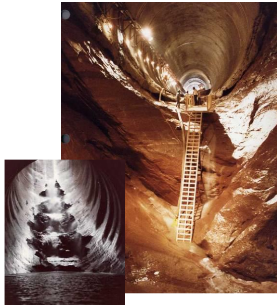
1983 Spillway Tunnel Damage due to Flood-induced Cavitation – Glen Canyon Dam, Arizona-Utah
