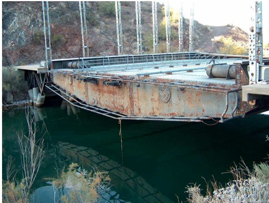
Parker Dam, Arizona: metal bulkhead for fixed-wheel mounted gate spillway
