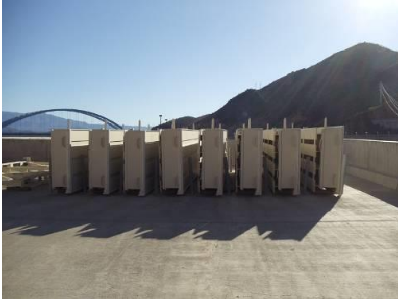
Theodore Roosevelt Dam, Arizona: metal stoplogs for top-seal radial gated spillways
