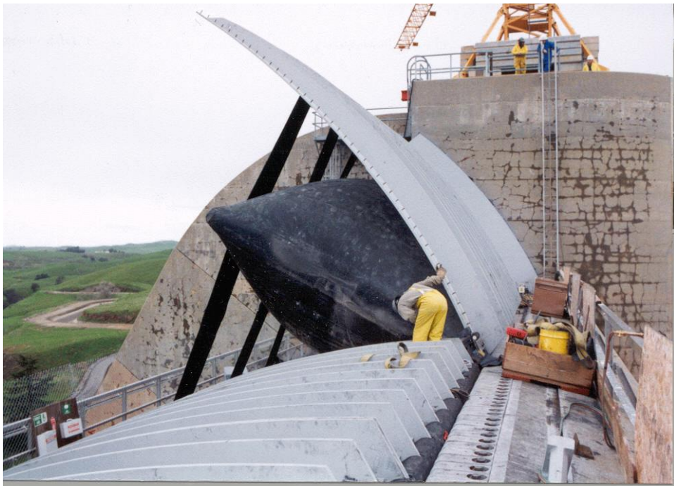
Figure 3.9.1.1-5. Crest gate – Obermeyer type.
