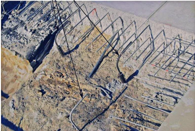
Scofield Dam, Utah: 2008-09 modification of existing spillway involving removing and replacing spillway chute slabs. Note installment of anchor bars into the rock foundation.
