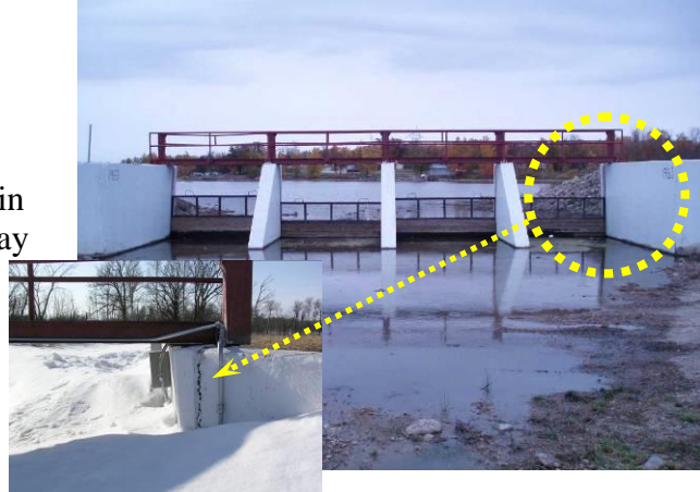
Spillway Walls Fail (concrete walls crack near base and reinforcement yields) due to Frost-Heave – Belcourt Dam, North Dakota
