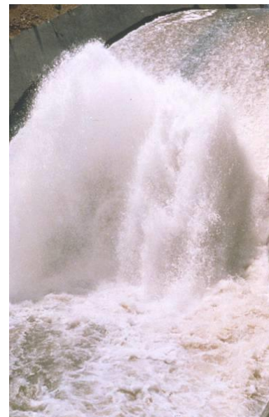
1983 Spillway Chute Damage due to Flood-induced Stagnation Pressure – Big Sandy Dam, Wyoming.
