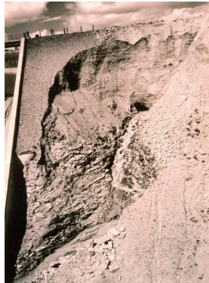
1965 Dam Internal Erosion Incident adjacent to Spillway during Normal Operations – Fontenelle Dam, Wyoming.
