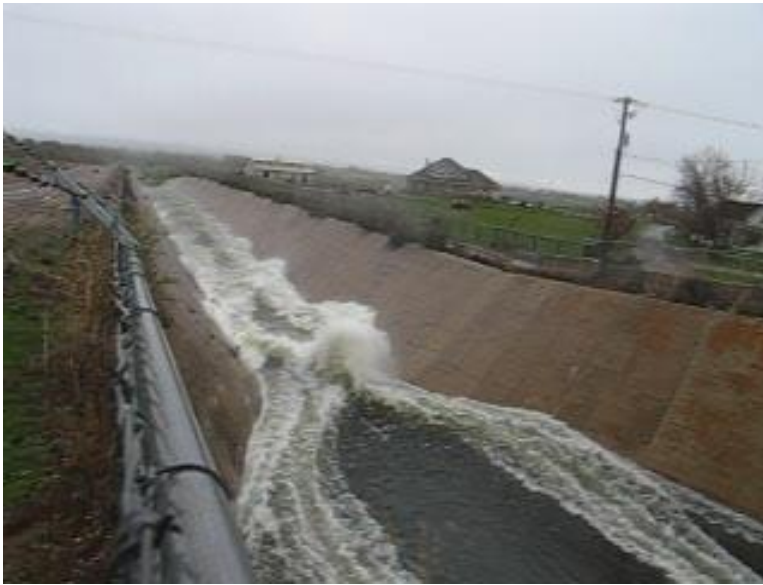
2005 spillway operation. Standing wave at downstream end of transition with cross waves downstream of standing wave – Hyrum Dam, Utah.
