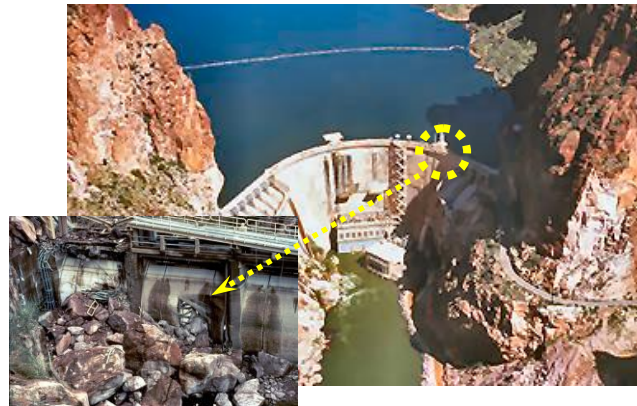
1992 Spillway Gate Damage due to Rockfall – Horse Mesa Dam, Arizona
