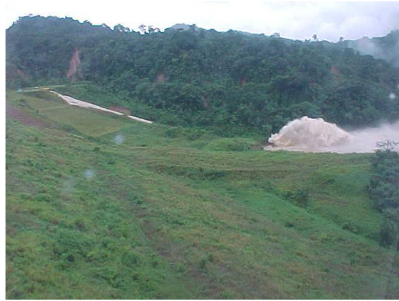
1999 Stilling Basin Sweepout (erosion in downstream channel creating “roster-tail”). Dam Failed due to Flood-induced Chute Wall Overtopping – El Guapo Dam, Venezuela (courtesy of Ing. Alejandro Hitcher).
