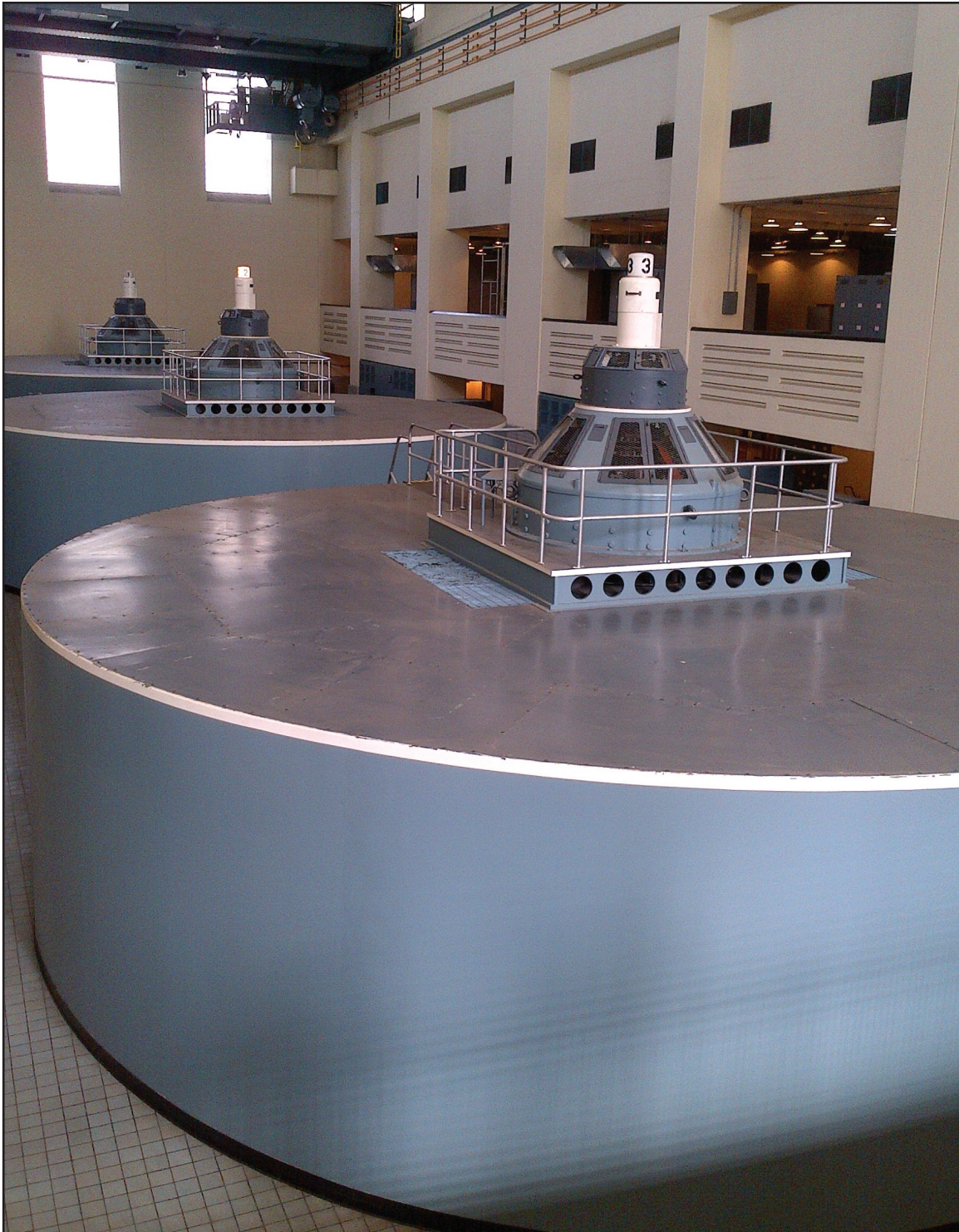
Customers approved funding of $26.9 million in FY 2013 to rehabilitate Center Hill powerhouse generators and turbines.
