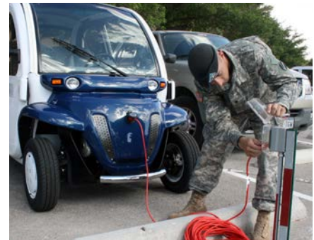
Figure 6-5. Spc. Dean Kalogris from Headquarters Company, Fort Bliss, Texas, charges the installation's command sergeant major's electric car using Level 1 charging equipment.
