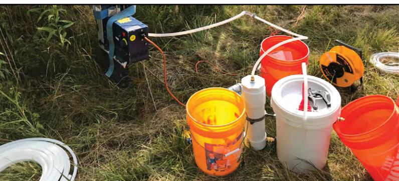
During this redevelopment of a well using a surge block, the purged water was filtered through activated carbon.
