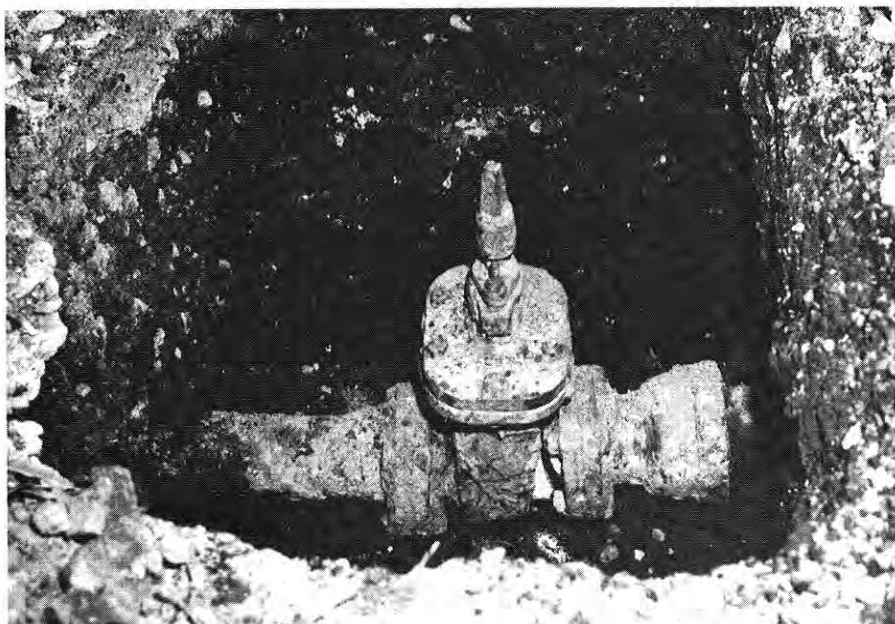
Figure 5.106a. Four-inch gate valve in water main broken by debris from brick wall (0.23 mile from ground zero at Hiroshima).
