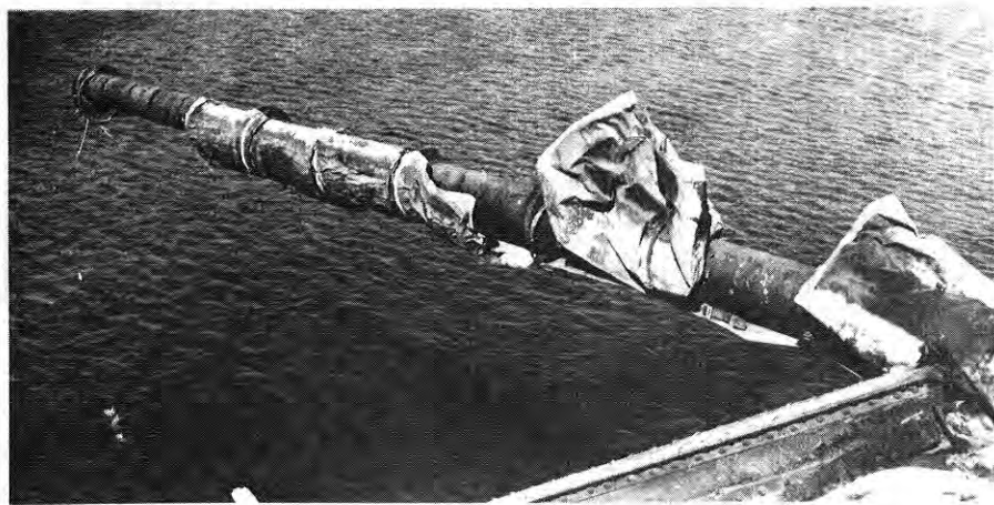
Figure 5.106b. Broken portion of 16-inch water main carried on bridge (0.23 mile from ground zero at Hiroshima).
