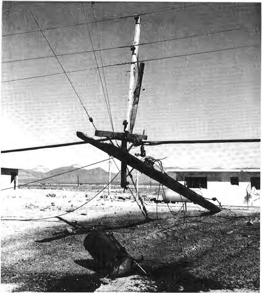
Figure 5.105. Transformer fallen from collapsed utility pole (5 psi peak overpressure), Nevada Test Site.
