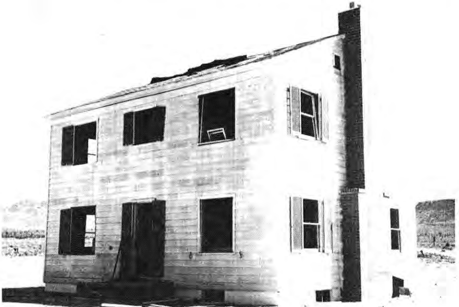
Figure 5.59. Wood-frame house after a nuclear explosion (1.7 psi peak overpressure).
