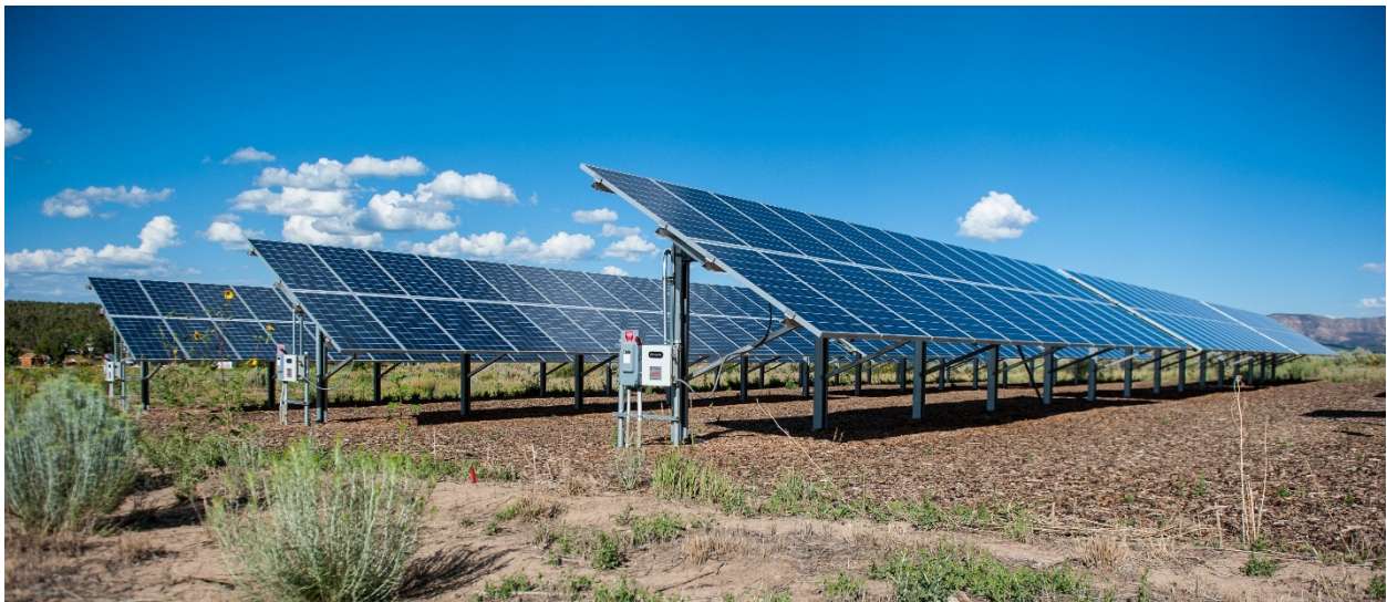
Figure 7. A ground-mount solar array using a dual pier support system
