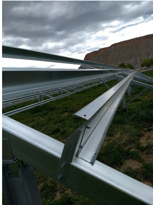
Figure 9. Cold rolled steel support structures are lightweight but can be weak along certain axes.
