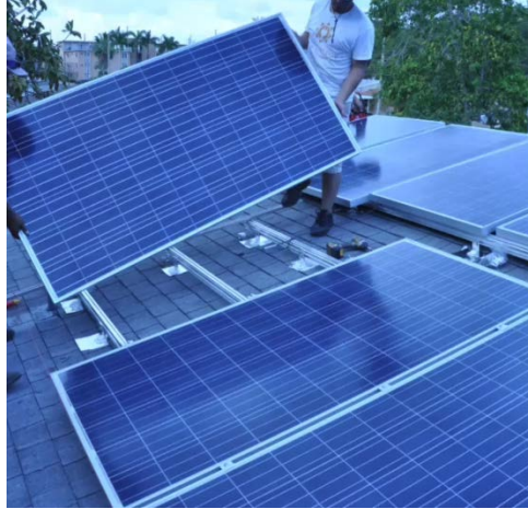
Figure 4. A solar installation in hurricane-prone Florida using a three-framed rail system to support the solar modules.
