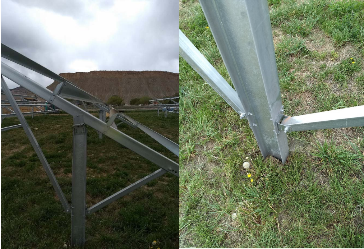
Figure 6. Solar PV racking with a single support pile.
