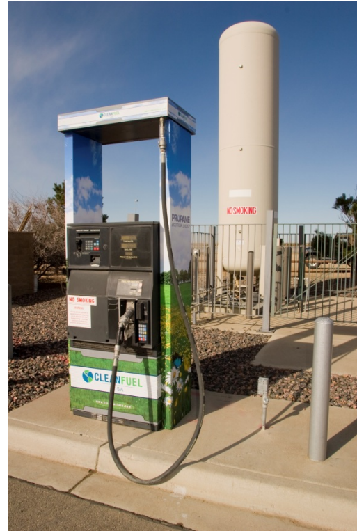
Propane dispenser and 2,000-gallon tank. Photo from CleanFUEL USA, NREL 28219
