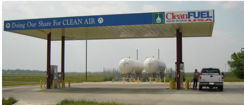
Austin-Bergstrom International Airport self-service propane station with twin 18,000-gallon tanks. Photo from CleanFUEL USA, NREL 28220
