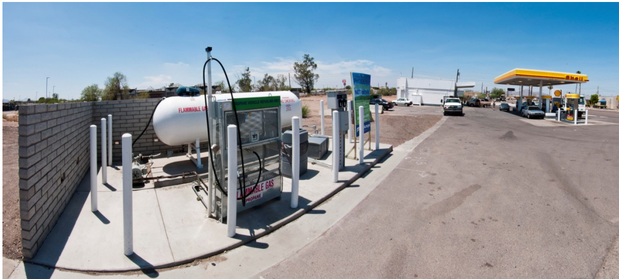
Propane station adjacent to a gasoline station in Phoenix, Arizona. Photo by Gabe R. DeWitt, NREL 30248
