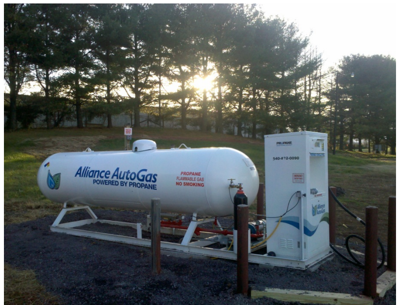
Skid-mounted 1,000-gallon propane storage tank and dispenser. Photo from Blossman Gas, Inc., NREL 30340
