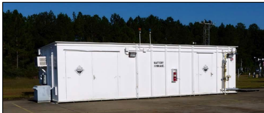
Figure 1-8. Battery Storage Facility (Building 3215)
