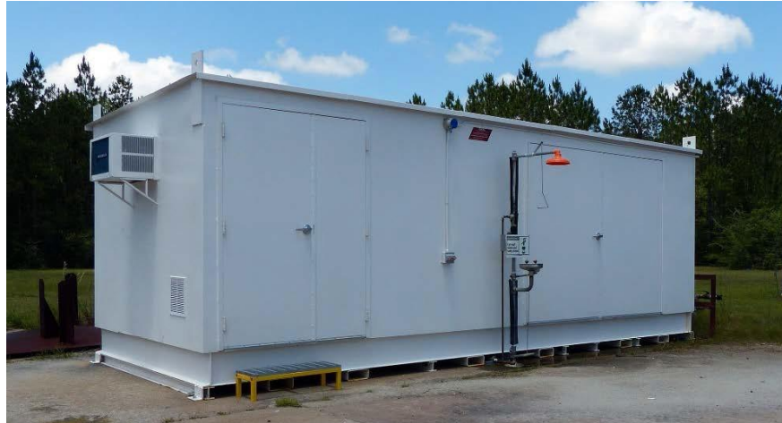
Figure 1-9. Lithium Battery Storage Locker (Building 3209-A)
