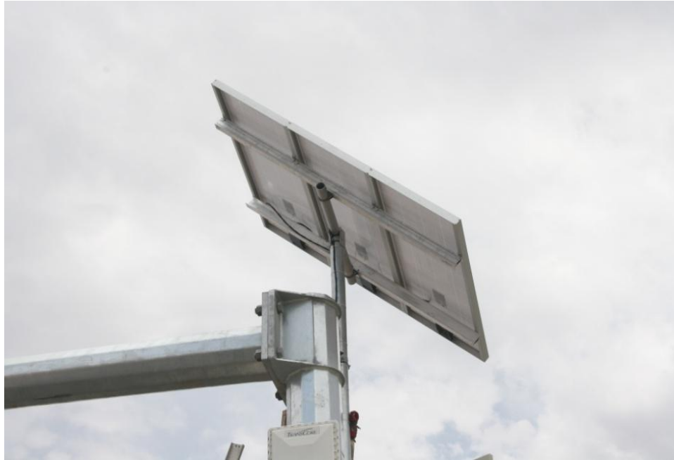
Figure 24. Photo. Solar panel installed at Ciudad Juárez, Mexico.
