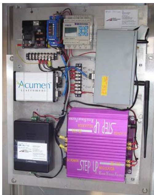
Figure 20. Photo. Back panel with communication hardware installed inside a cabinet as part of the RFID reader station.
