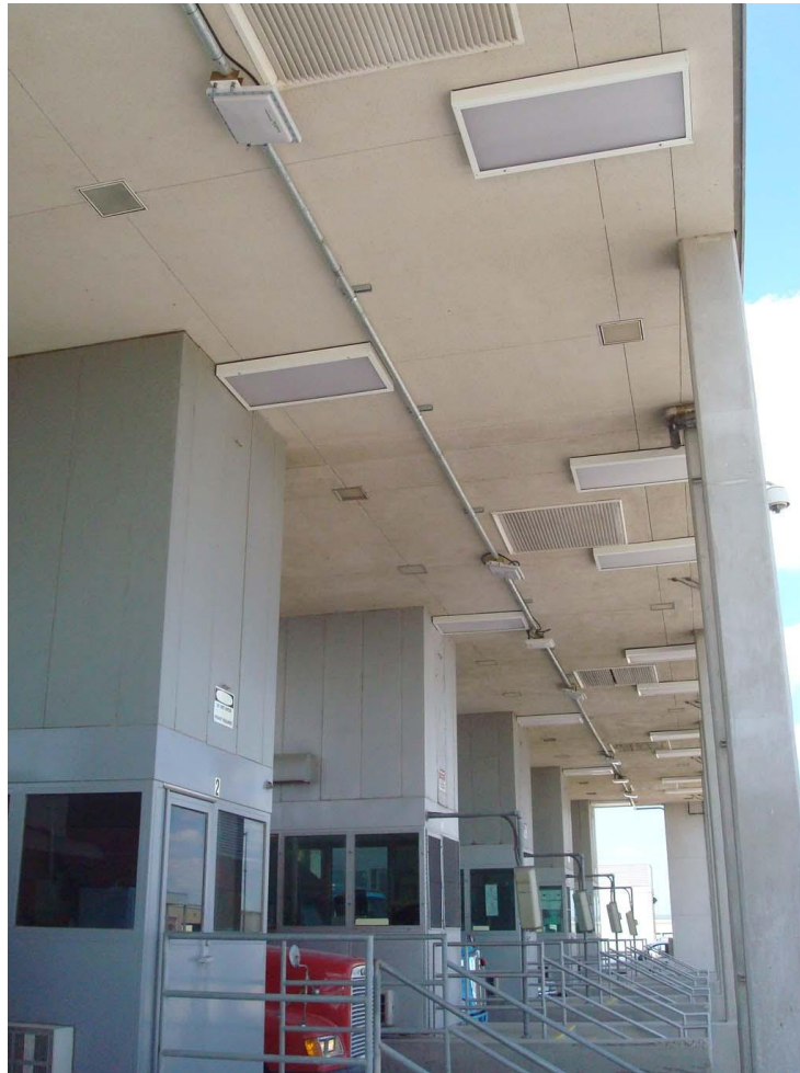
Figure 36. Photo. Installed RFID equipment at CBP's primary inspection facility at Pharr-Reynosa border crossing.
