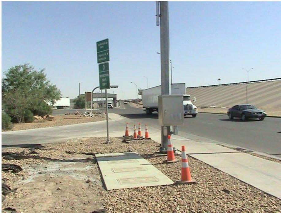
Figure 27. Photo. Power cabinet and in-ground battery installed at El Paso, US.
