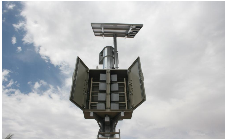
Figure 25. Photo. Pole-mounted batteries installed at Ciudad Juárez, Mexico.
