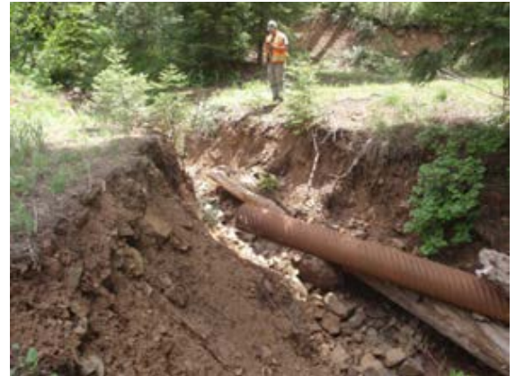
A crewmember examines a collapsed stream crossing in Idaho as part of GRAIP's forest road inventorying process.
