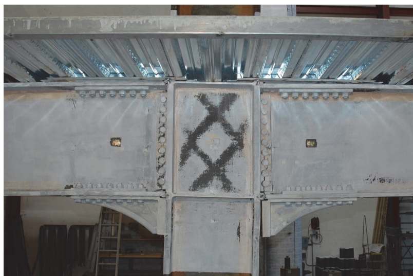
Figure 2-8 Shear buckling of thin doubler plate in a retrofitted moment connection (Newell et al., 2006).
