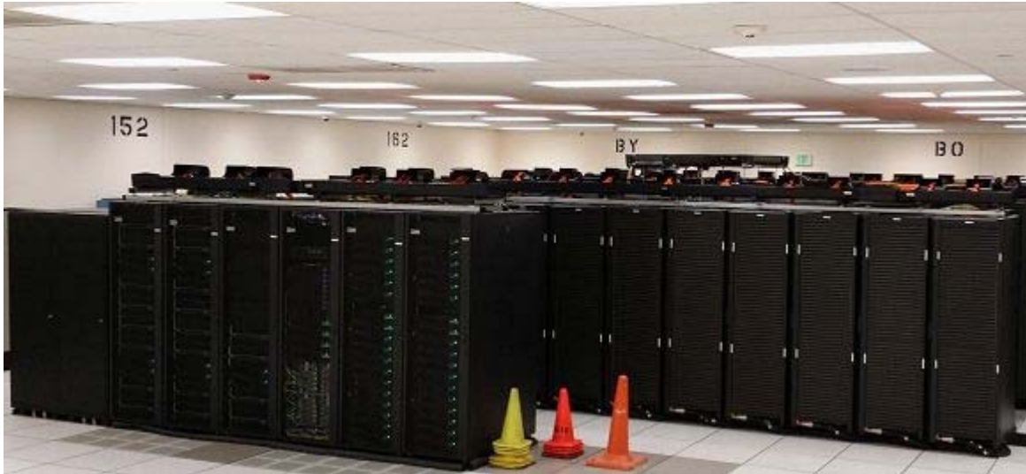
Picture of WCOSS Gyre (Phases 1 and 2) located in Orlando, Florida.
