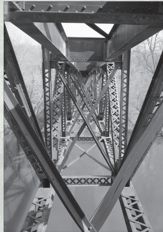
Western Maryland Railway, Cumberland Extension, Bridge No. 1396, Fourth Potomac and Second B&O Crossing, Maryland, Jet Lowe, photographer, 2010. HAER often works with national parks to document their historic engineering resources, such as the Western Maryland Railway, part of Chesapeake & Ohio Canal National Historical Park.
