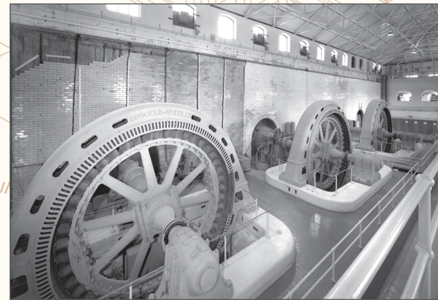
Chicago Sanitary and Ship Canal, Lockport Power House and Dam, Lockport vicinity, Illinois, Jet Lowe, photographer, 2009. Crocker-Wheeler generators remain in the Lockport Power House on the Chicago Sanitary and Ship Canal.
