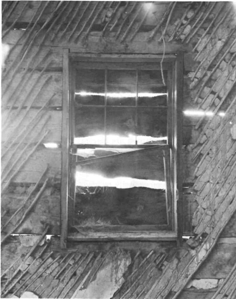
Log cabin No. 2, Spring City, Utah. A rare and interesting structural detail: the use of vines for lath.
