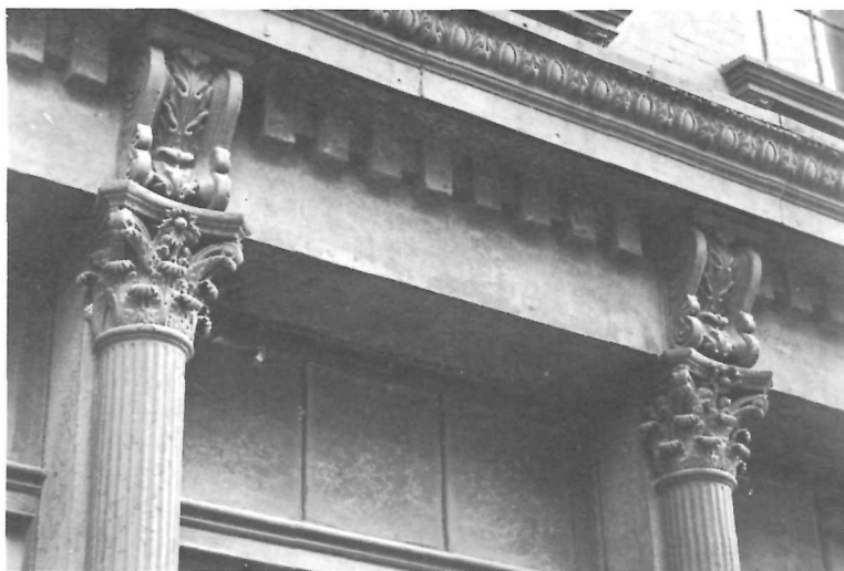
Building, 9 North Commerce St., Mobile, Ala. This photograph gives a detailed record of the cast-iron columns and entablature.
