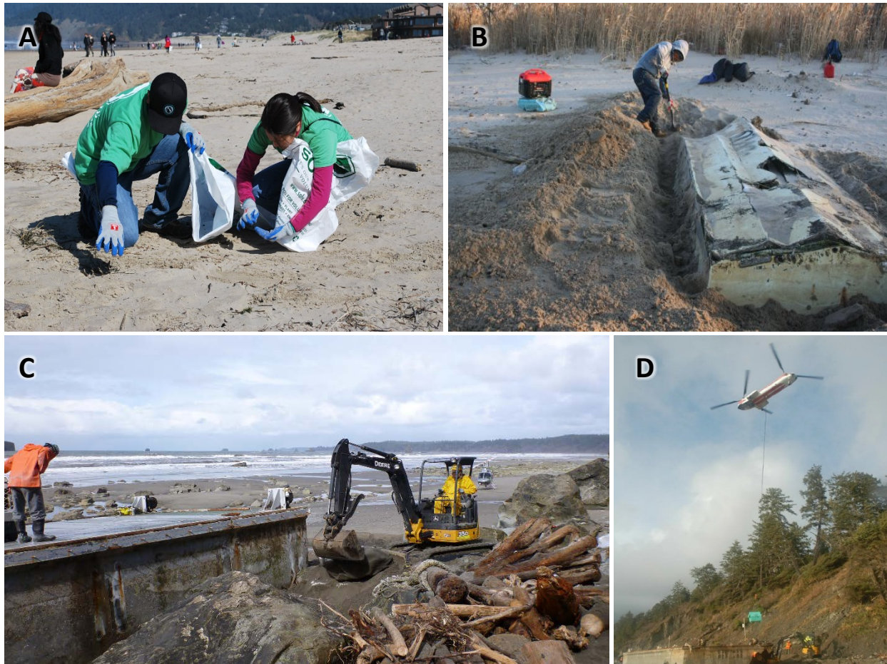
Figure 5. Examples of equipment and removal methods suitable for removal of debris items on un-vegetated intertidal substrates such as beaches and flats including manual removal (A), manual removal with limited hand excavation (B), use of small tracked equipment to assist in dismantling large debris item (C), and removal of debris components by helicopter sling load (D). Photo credits: American Littoral Society, WA Dept. of Ecology, NOAA MDP, and The Undersea Company.
