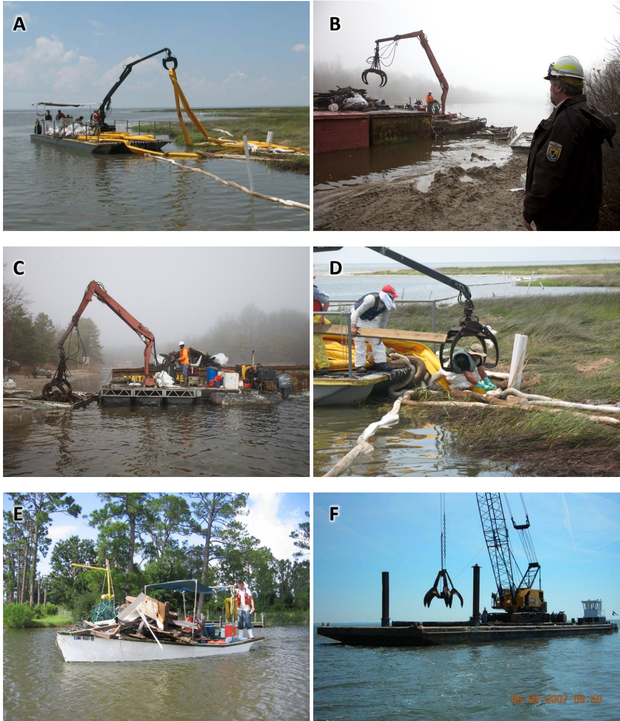
Figure 2. Examples of equipment and removal methods suitable for removal of debris items on edge or fringe of vegetated wetlands including boom-mounted grapple on shallow draft barge (A-C), detail of combined manual and grapple removal (D), small boom crane on vessel of opportunity (E), and large crane mounted grapple on barge (F). Photo credits: RPI, USCG, NOAA MDP, USFWS.
