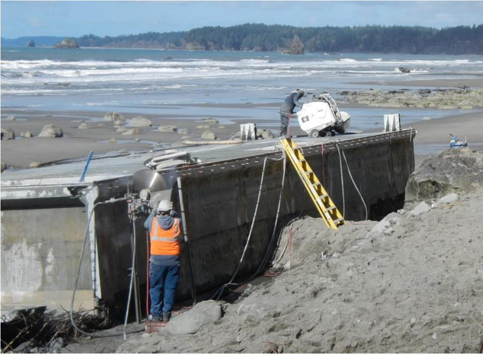
Figure 6: Cutting the Misawa floating dock that washed up at Olympic National Park, Washington, in December 2012. (NOAA)
