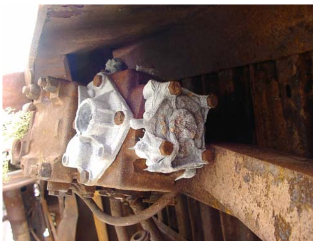
Figure 6-1. Air Brake Valve Found 20+ m [66 ft] from Fuel Spill Site (Note Only Partial Melting at This Location)
