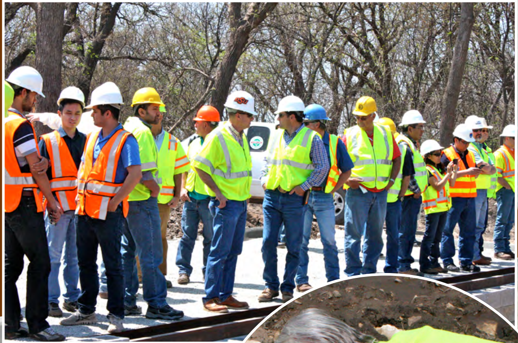
Transportation professionals observed as crews placed abutment layers at a GRS-IBS demonstration showcase in Oklahoma.
