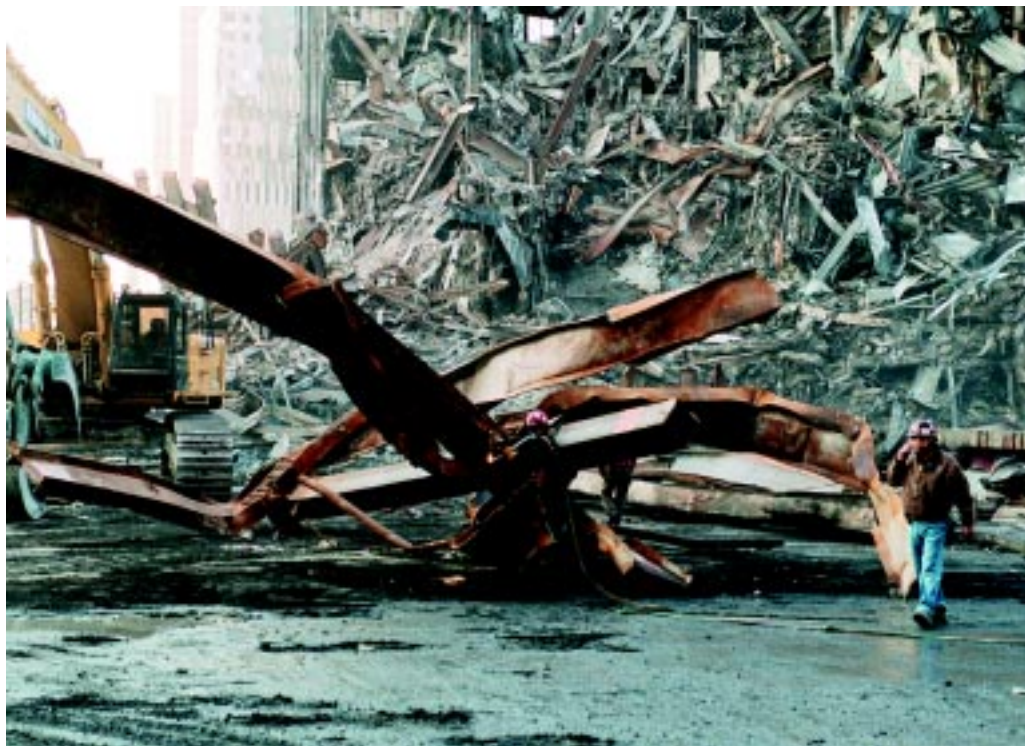
Twisted steel and other debris at the site posed many potential safety hazards.
