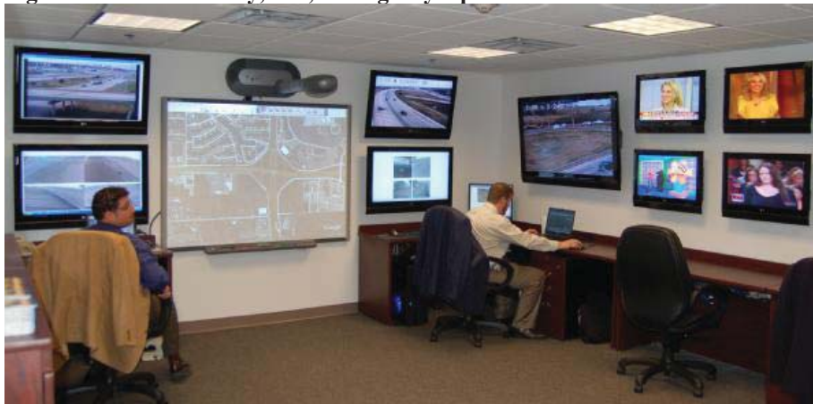
Figure 3. Oklahoma City, OK, Emergency Operations Center
