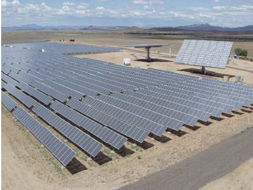
Figure 5.2.1. Arizona Public Service's Prescott Airport Solar System Showing a Tracking Flat-Plate, Nonconcentrating PV System. In the background are concentrating PV systems. (Source: Herb Hayden, Arizona Public Service)
