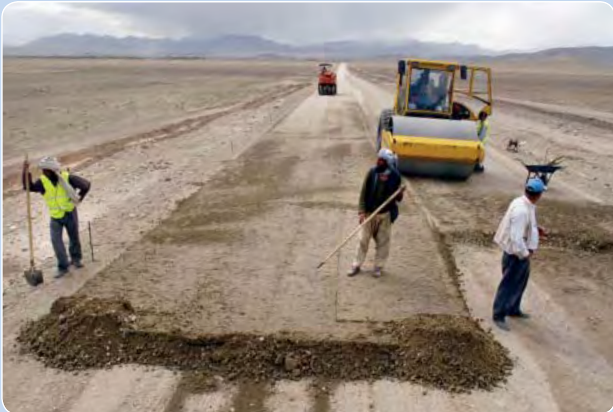
Workers build a road from Ghazni to Gardez, linking the region to the main highway connecting Kabul to major cities.
