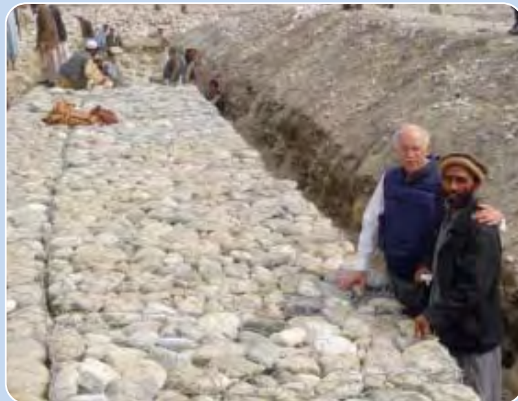
USAID Administrator Natsios with head engineer Askar in Muftie, Rodat (Nangarhar), Afghanistan. Building gabion walls and removing 25 years of built-up silt from the canals will significantly increase the flow of water to the affected area, enabling farmers to grow crops needing multiple floodings. PHOTO: USAID/MICHELLE PARKER
