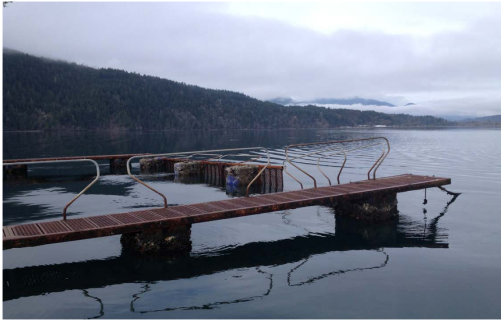
Broken net pen at Skokomish hatchery
