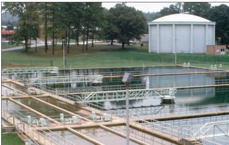
Chattahoochee Water Treatment Plant, City of Atlanta, Georgia. Photo by Nancy L. Barber, USGS.
