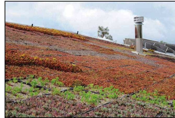
A modular extensive green roof in Fallbrook, California, was installed on the roof of a public library. Prefabricated plastic trays were planted with colorful varieties of stonecrop.
