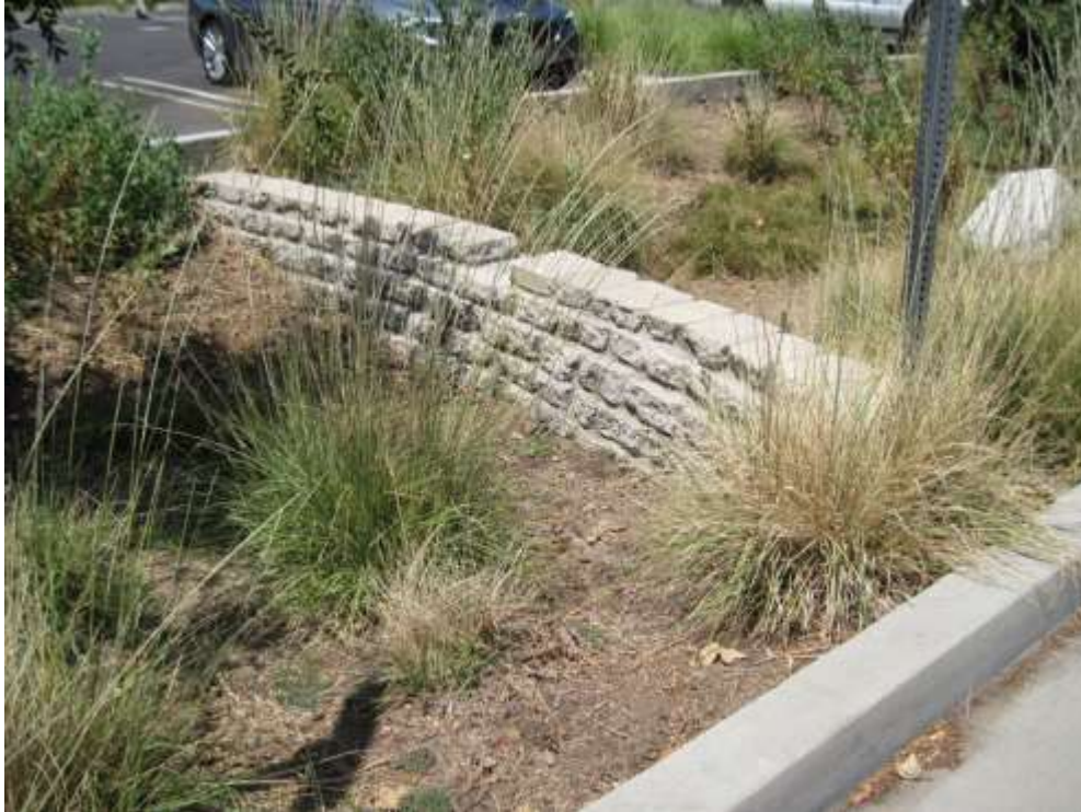
Los Angeles, California. Source: Tetra Tech Figure B-2-4. Bioswale with a check dam.
