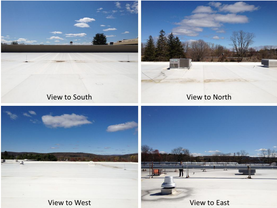
Figure 8. Views of the feasible area for roof-mounted PV on Building 52 at the TechCity East Campus. Photos by James Salasovich, NREL
