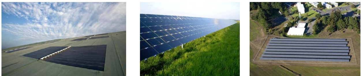
Figure 4. Thin-film solar panels installed on a (left) solar energy cover and (middle/right) fixed-tilt mounting system. Photos by (left) Republic Services, NREL 23817, (middle) Beck Energy, NREL 14726, and (right) U.S. Coast Guard Petaluma Site, NREL 17395
