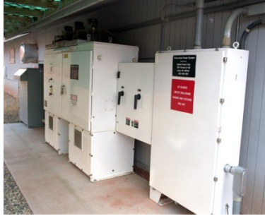
Figure 5. String inverter. Photo by Warren Gretz, NREL 07985
