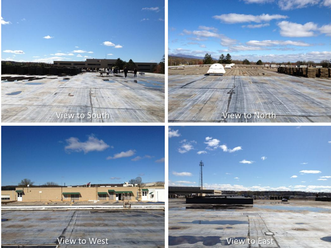
Figure 7. Views of the feasible area for roof-mounted PV on Building 1 at the TechCity East Campus. Photos by James Salasovich, NREL
