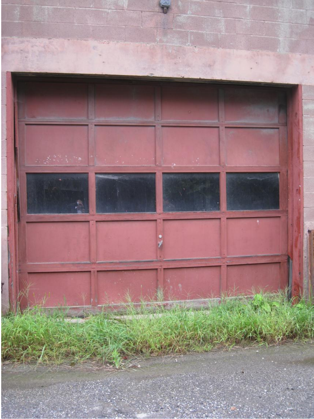
Figure 12. Large roll-up door on a site building. Photo by Randolph Hunsberger, NREL
