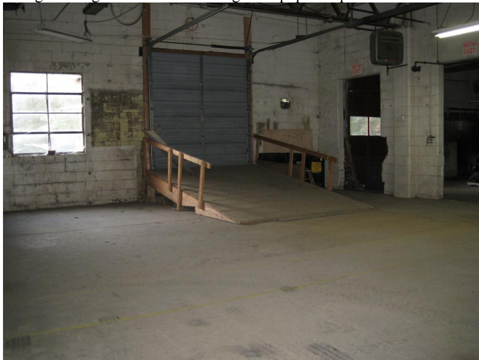
Figure 10. Inside a site building with large delivery doors. Photo by Randolph Hunsberger, NREL
