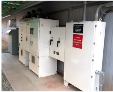
Figure 5. String inverter. Photo by Warren Gretz, NREL 07985
