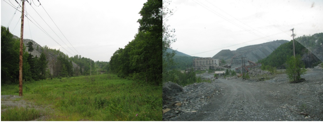
Figure 11. Electrical tie-in point for the PV system (left) and site distribution (right). Photos by Joe Simon, NREL
