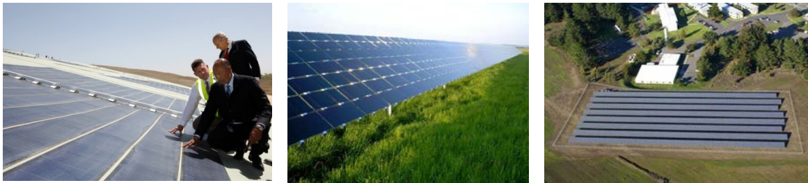
Figure 6. Thin-film solar panels installed on (left) solar energy cover and (middle and right) fixed-tilt mounting system. Pictures from (left) City of San Antonio, NREL 18068; (middle) Beck Energy, NREL 14726; and (right) U.S. Coast Guard Petaluma site, NREL 17395
