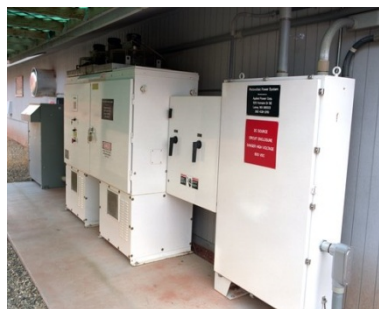
Figure 7. String inverter. Photo by Warren Gretz, NREL 07985
