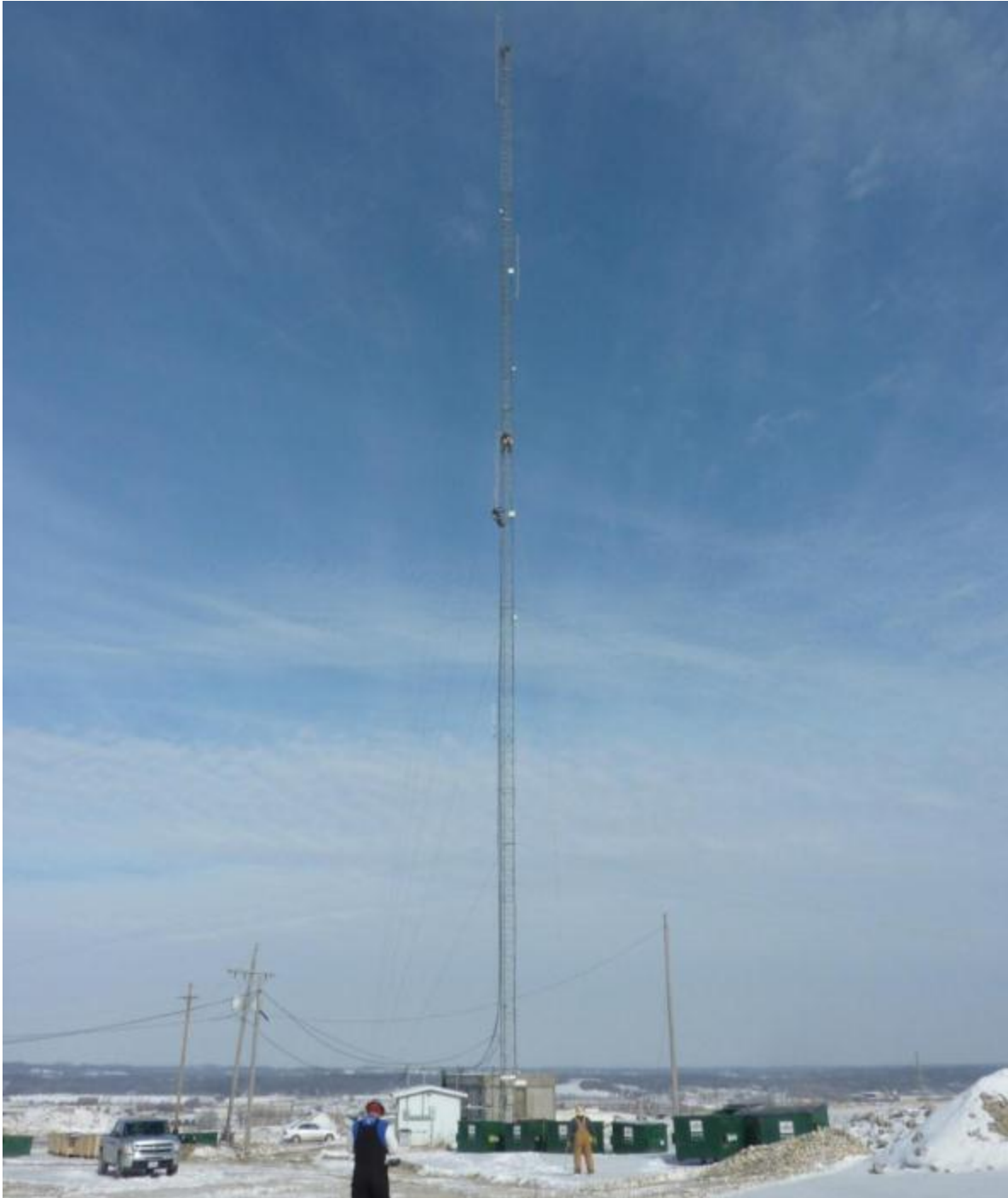
Figure 10. Riggers installing anemometry on the Doepke tower. Photo from Shelly Brodie, EPA
