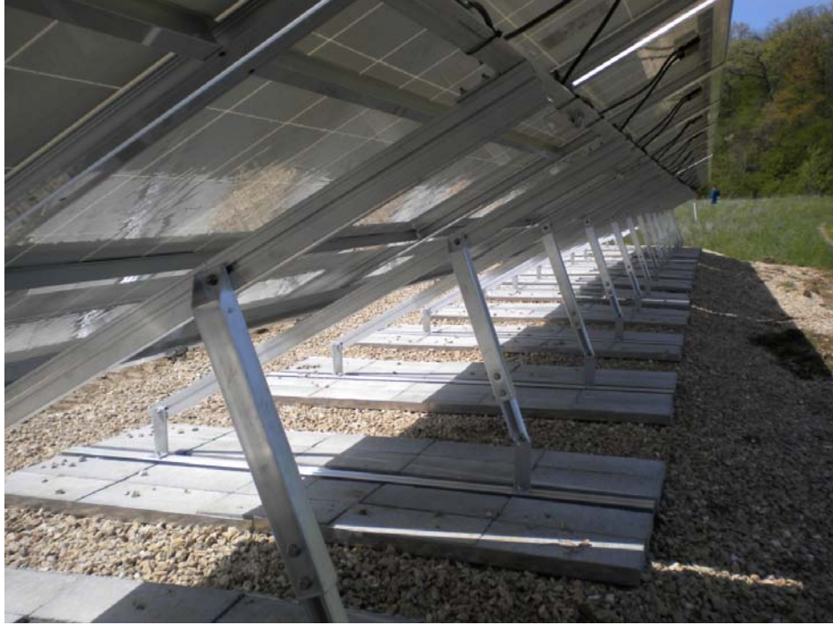
Figure 4. Ballasted PV system at the Refuse Hideaway Landfill
