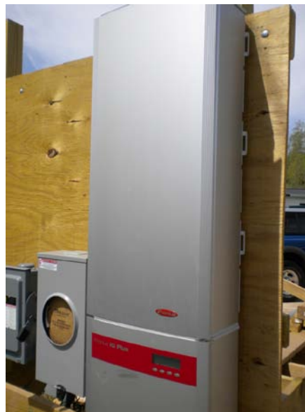
Figure 7. Inverter used in the PV system at the Refuse Hideaway Landfill
