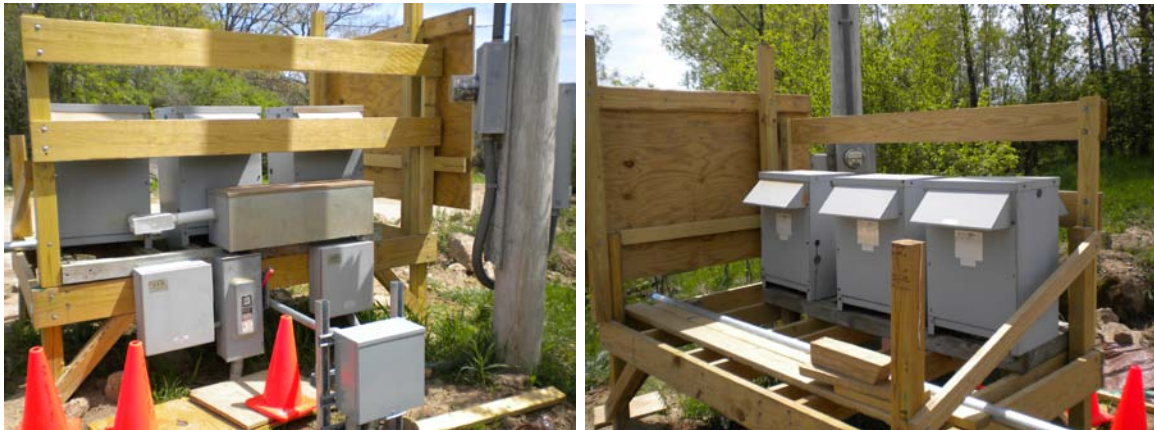
Figure 6. Electrical tie-in point for the PV system at the Refuse Hideaway Landfill
