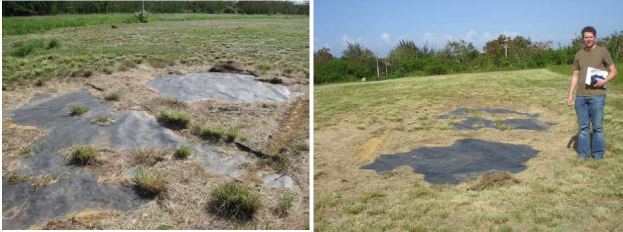
Figure 6. Views of the exposed impermeable plastic liner of the Cataño Landfill cap
