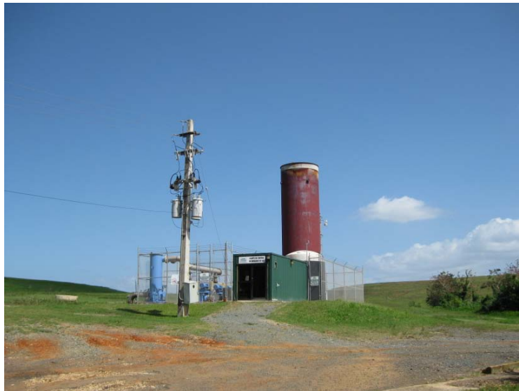
Figure 20. San Juan Landfill gas flaring facility
