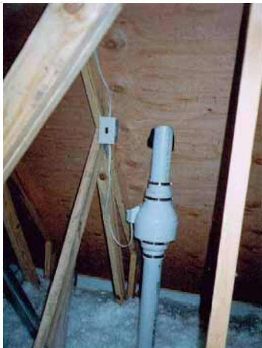
Figure IV-4: Fan in Attic
