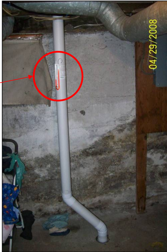
View of the extraction well pipe inside the basement.
