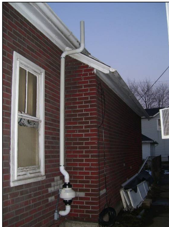
View of the outside fan and the piping which vents the vapors that accumulate beneath the property
