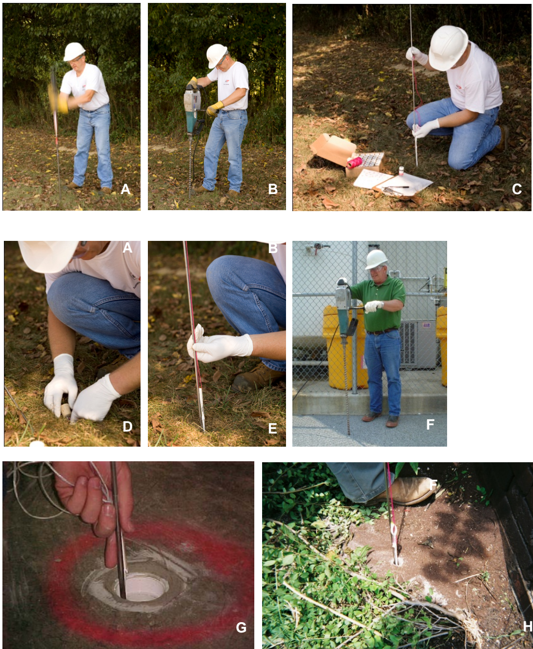
Figure F12. Passive soil vapour module installation. Photos A to E: Exterior soil vapour sample using slide hammer and rotary hammer drill, insertion of a passive soil gas sampler, and sealing hole. Photos F to H: Subslab soil vapour sample.
