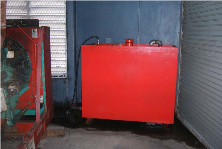
Photo description: Oil tank for generator in LC-3, not located inside the oil retaining wall
