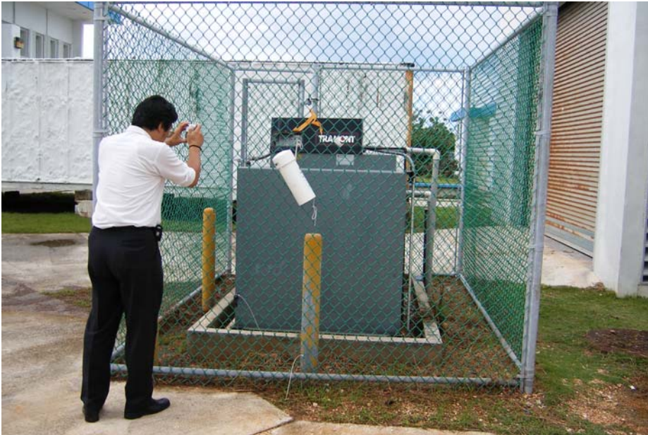
Photo description: Oil tank for LC-1
