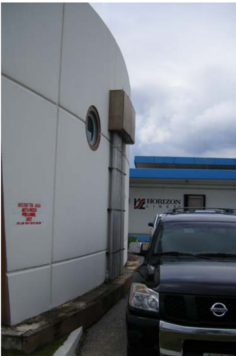
Photo description: Cable pipes outside LC-1
