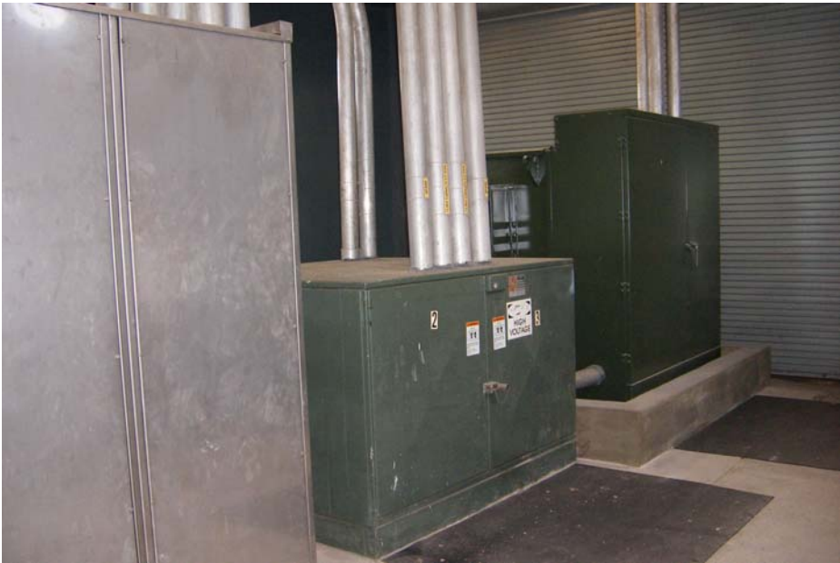
Photo description: Switchgear and transformer in LC-1
