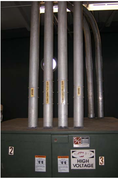
Photo description: Outgoing HV cables from LC-1 to LC-2 and LC-3
