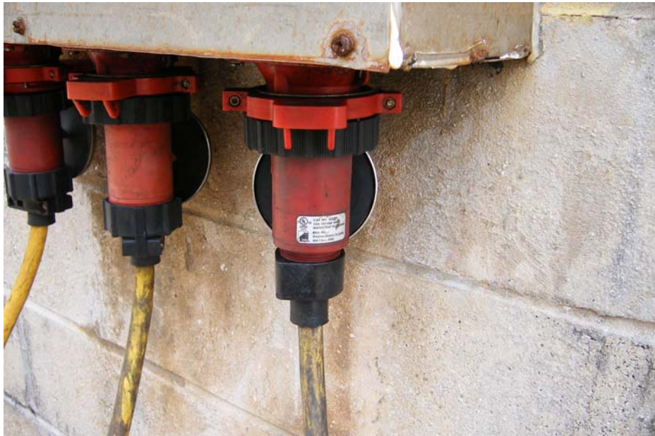
Photo description: Close up view of reefer socket outlet
