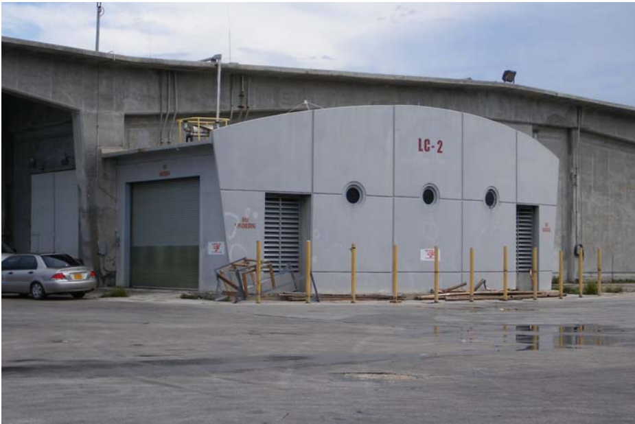
Photo description: Load Center (LC #2)
