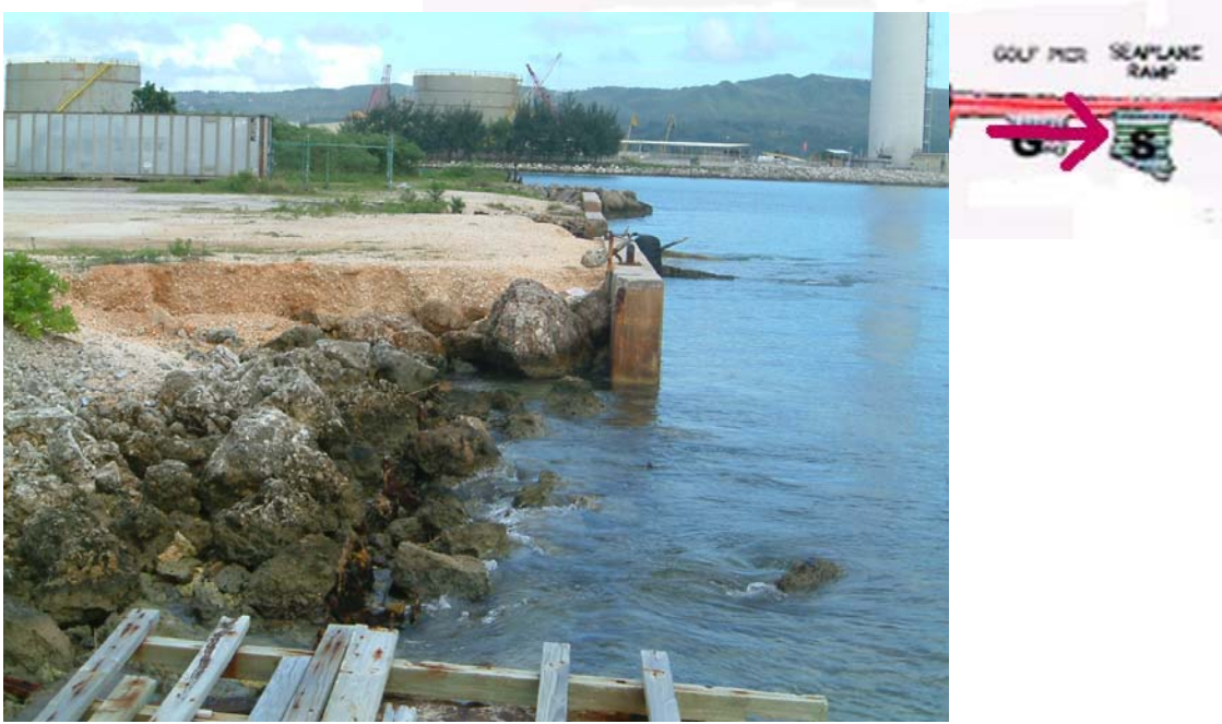
Photo description: A close up view about the damage from the land side in the left side of the Seaplane Ramp
