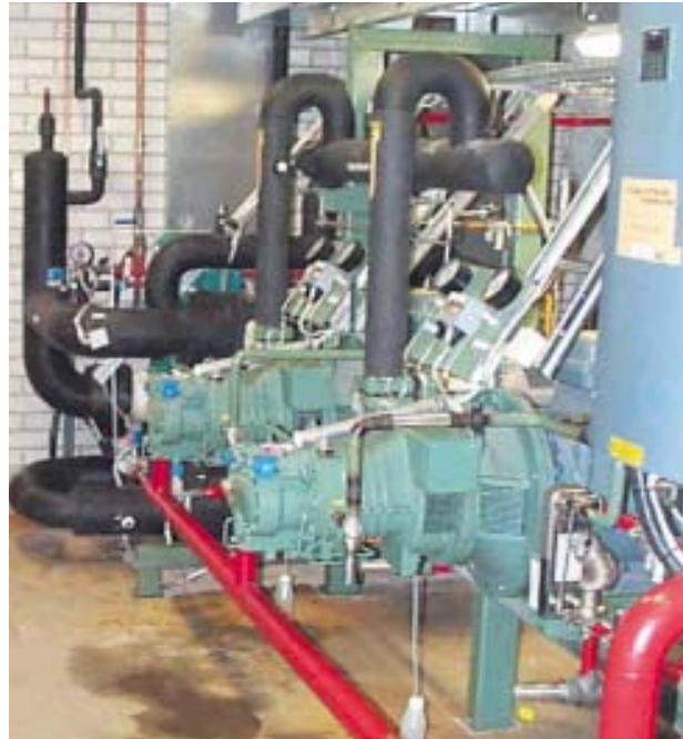
Figure 13. Two screw compressors.
