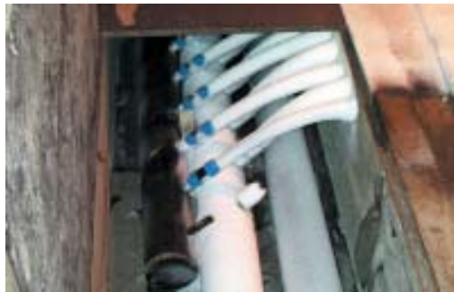
Figure 12. Plastic rink piping connections to the distribution and the collection mains (thermally insulated).
