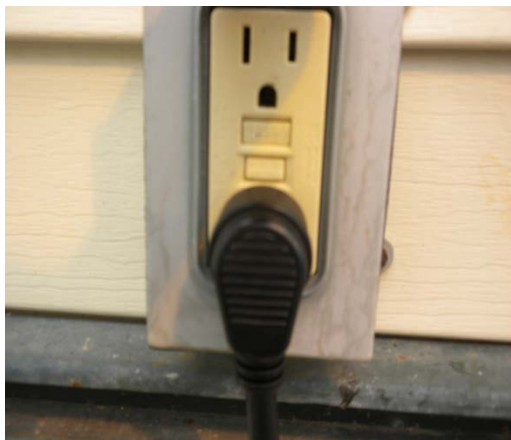
Figure 12. GFCI outlet as electricity source
