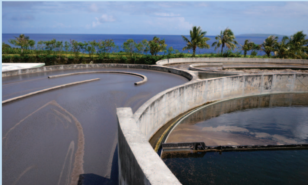
EPA helped fund construction of this wastewater treatment plant in Saipan.
